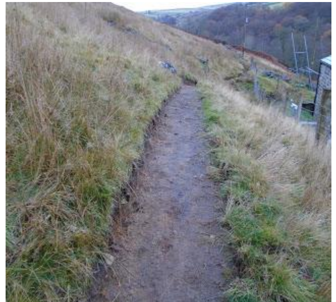
We completed improvements on the paths that run down from the tops into Hardcastle Crag – cutting back, widening, drainage and stiles.
